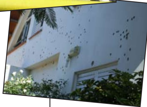
Rocket damage near the Zadok's house
